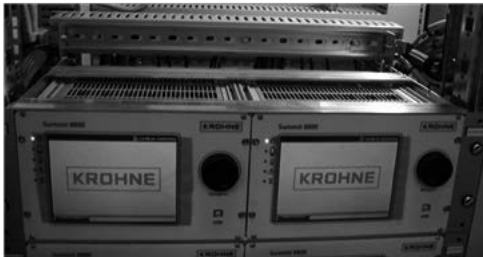
Figure 9 Rack mounted installation
