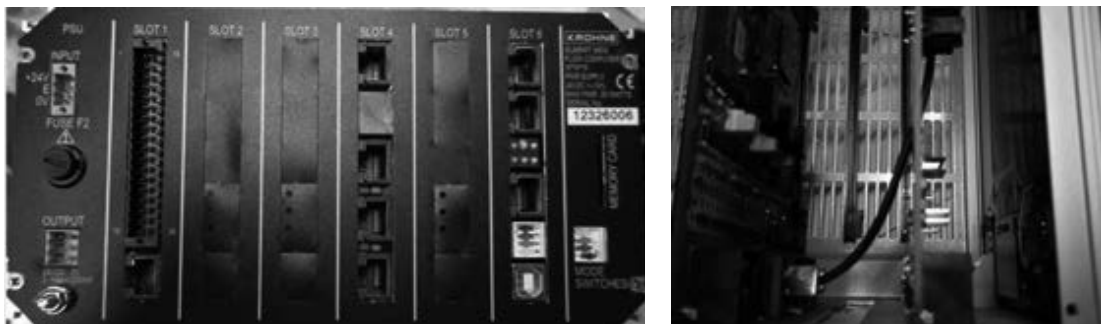
Figure 52 DSfG communication installation
